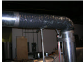
Fig. 2 Test w/ kinked duct
